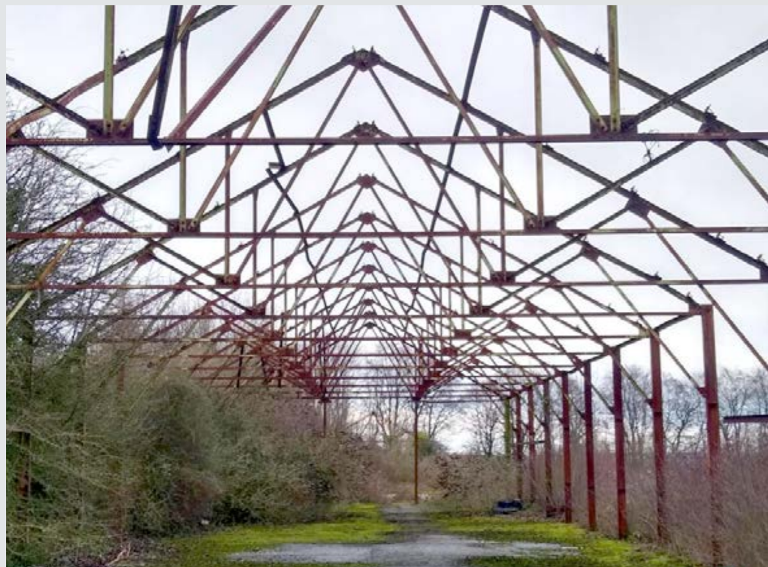
Remaining steel frame which formed part of the Camp's Gymnasium building.
